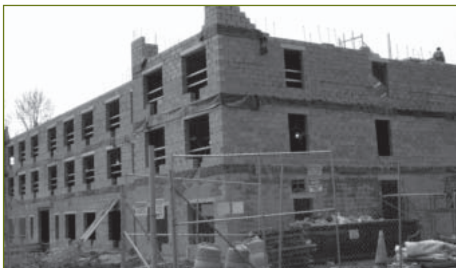
Ludlow House is rising on Riverdale Avenue in Yonkers, approximately halfway between St. Joseph's Medical Center and St. Peter's Church.
